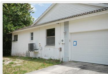
A home that has a code violation sticker attached.
